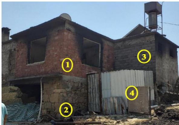
Figure 16: Damages in the mixed materials (four types of materials)
