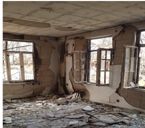
Figure 10: Inside spalling of plaster
