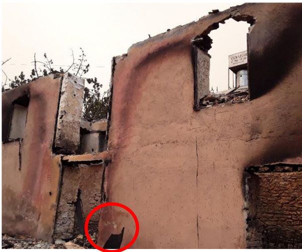
Figure 9: Spalling of plasters in the facade
