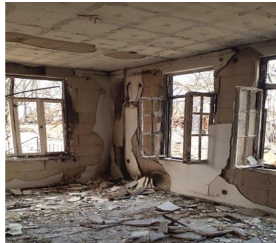
Figure 10: Inside spalling of plaster
