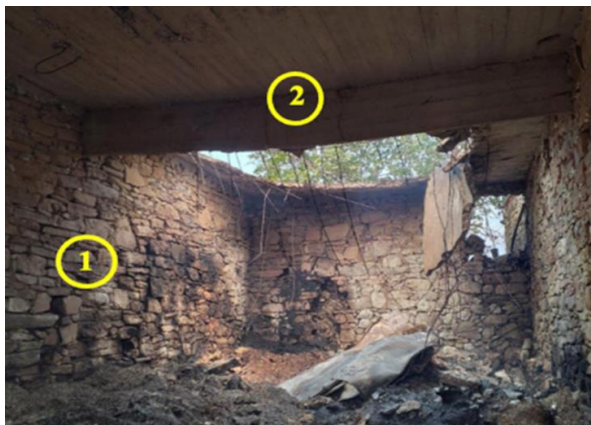
Figure 17: Damages in the mixed materials (two types of material)
